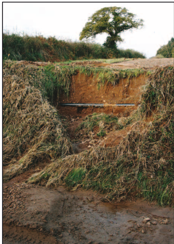
Figure 16. Damage caused by water flowing out of fields and over the earth banks lining the road running south towards Fluxton on the western side of the Otter Valley. Note the exposed utility pipe. The width of the hole is approximately two metres.
